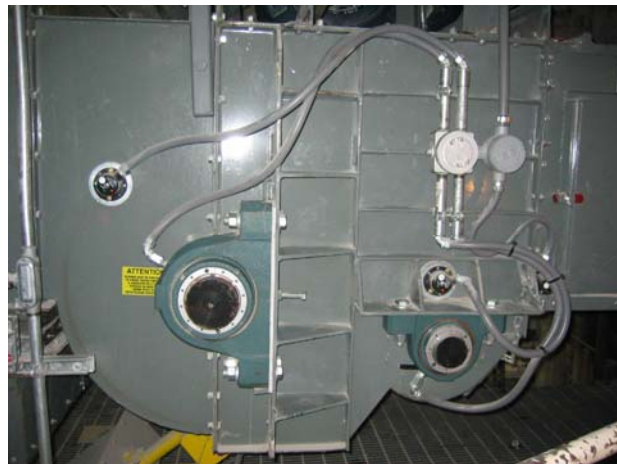
Figure 16. Force activated belt misalignment switches installed on enclosed belt conveyor
