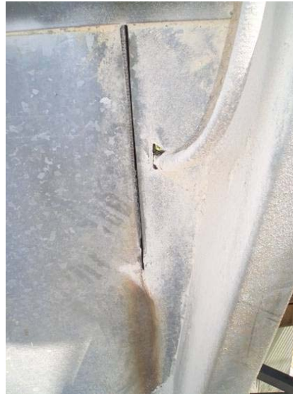
Figure 13. Outside elevator casing showing slit in steel casing and heat build-up due to severe belt misalignment
