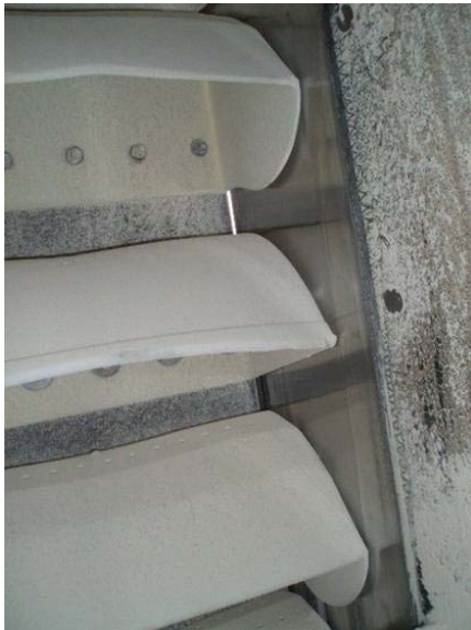
Figure 12. Inside elevator casing showing slit in steel casing due to severe belt misalignment
