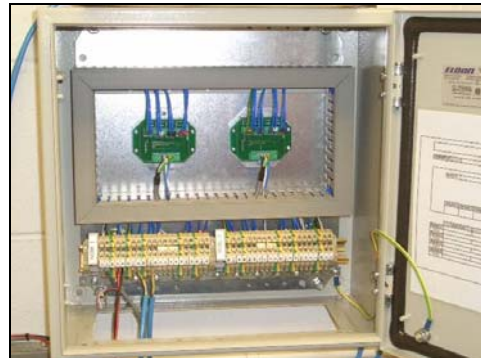
Figure 28. Good wiring installation
